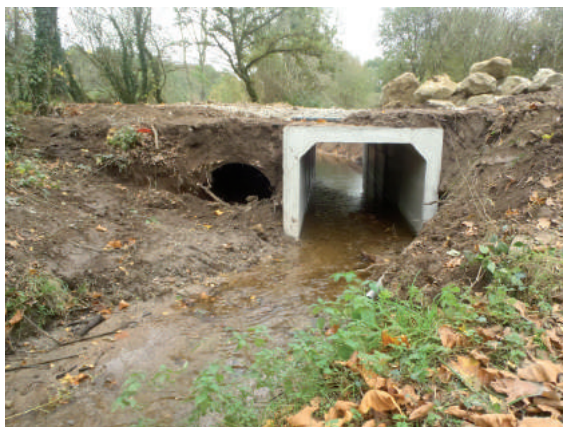
Replacement of an undersized metal culvert (left) by a rigid-frame bridge (right) on the Bonne Chère.
