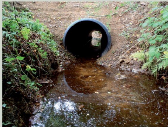
Replacement of a narrow culvert—an impassable barrier to fish—with an Ecopal plastic tunnel on an affluent of the Loc'h.
